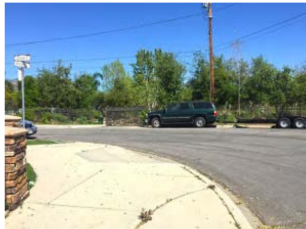
Ramp missing truncated domes for visually impaired users at Eighth Street and Newton Street
