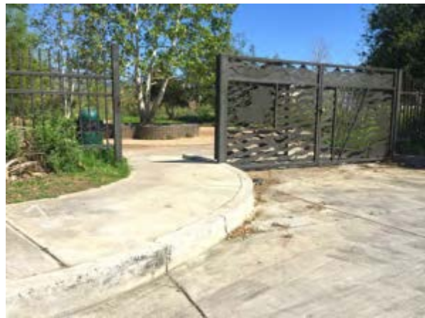
Missing curb ramp and truncated domes at entrance of Pacoima Wash Natural Park
