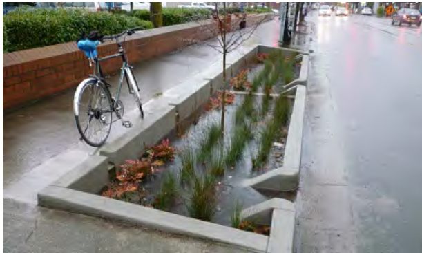
Curb cut-outs in depressed tree well/parkway allow water to seep in, be stored, and cleaned through system
