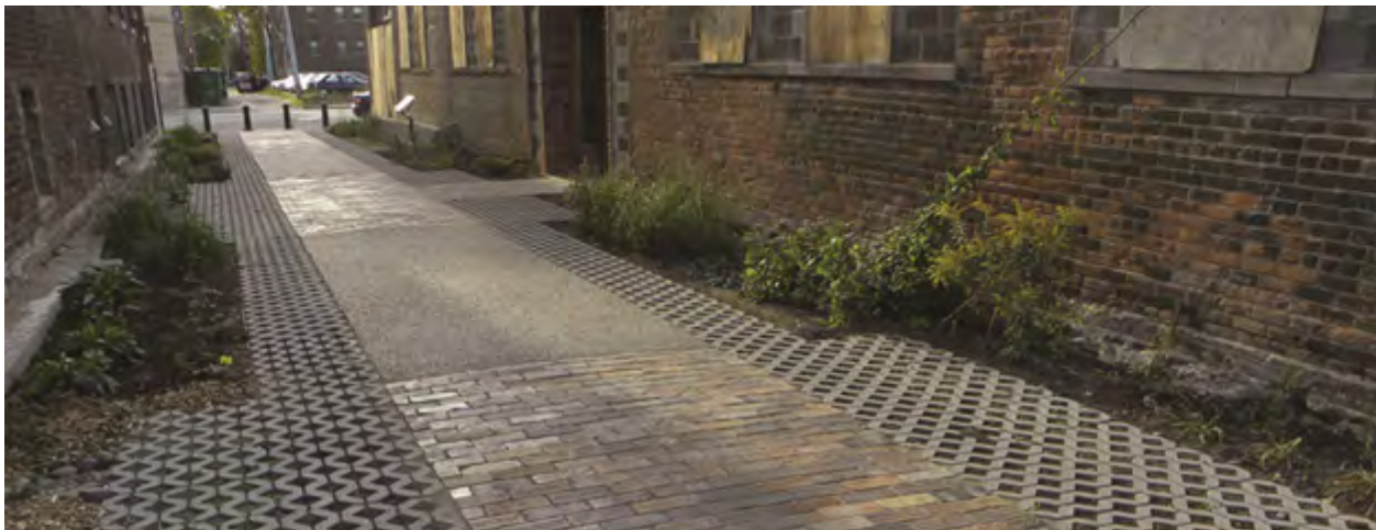
Green Alley uses bricks and permeable pavers to create a more inviting walking space and recapture water
