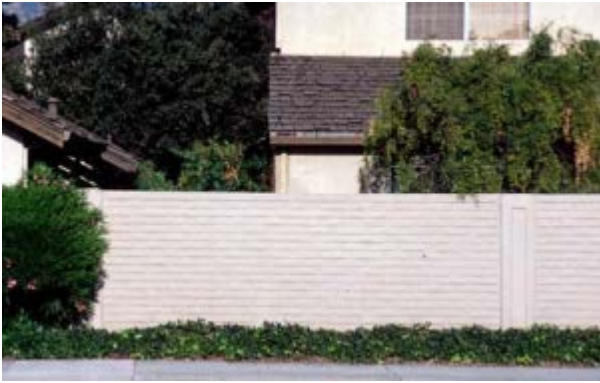
Plain block walls should NOT be used.
